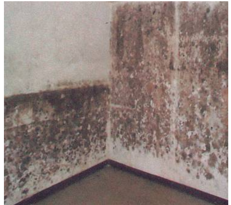
Mold growth on gypsum board from capillary action after flood
