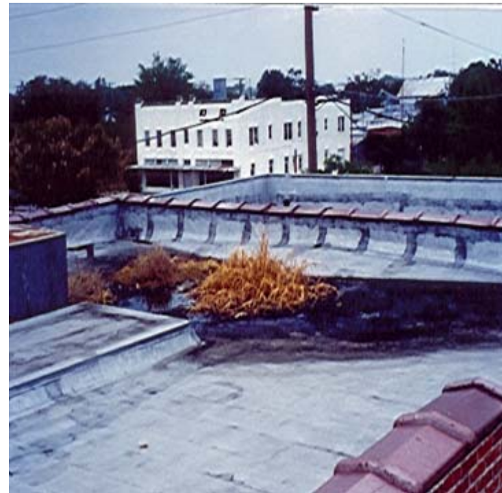
Unintended rooftop pool and garden
