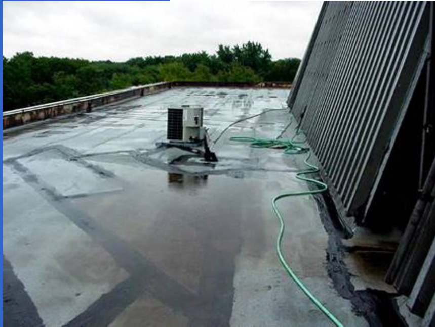
Improper drainage can result in severe water damage
