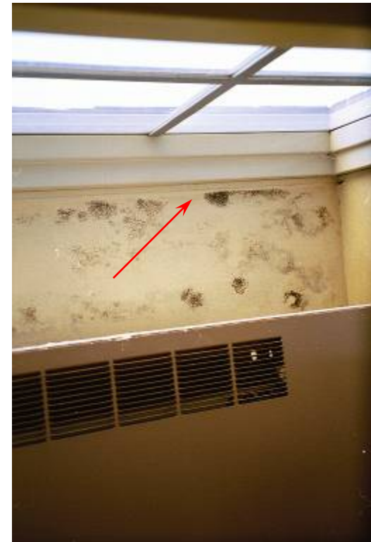
Mold resulted from poor window sealant
