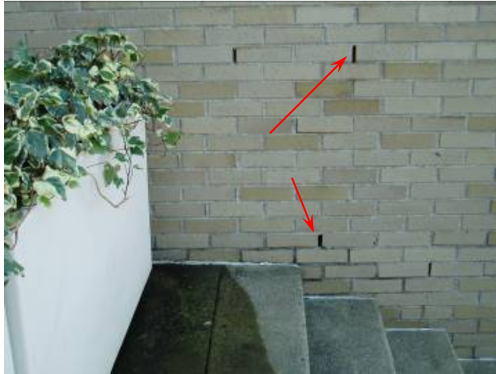
Missing mortar provides points of water entry
